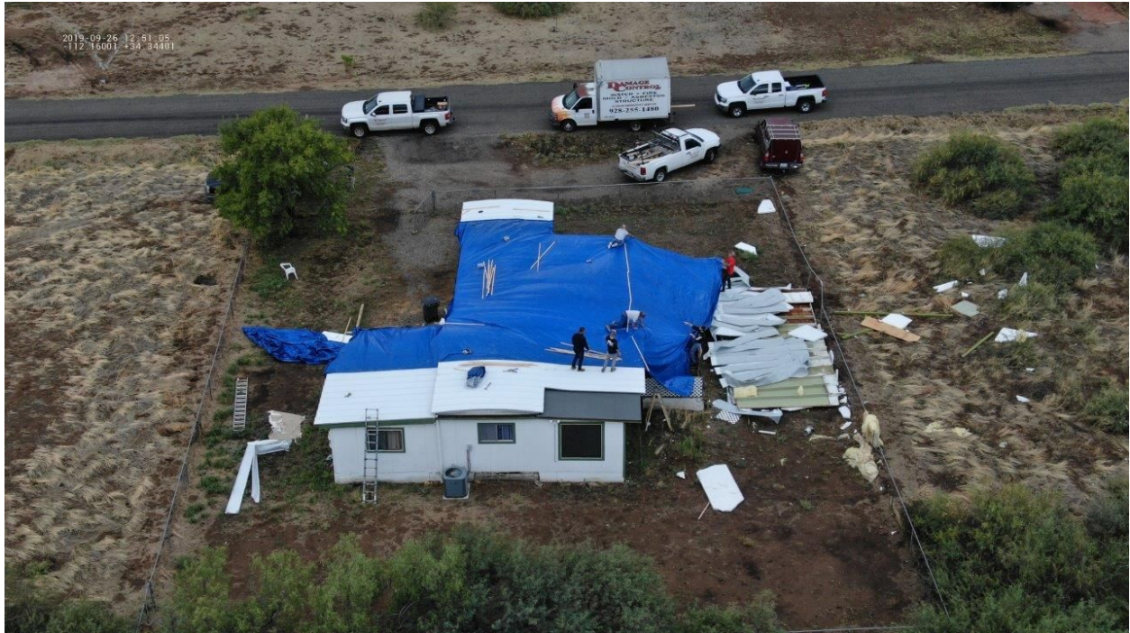
Image D - Storm Damage
